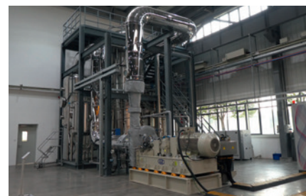
PILLER's falling-film evaporator in Taicang, China
