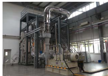
PILLER's falling-film evaporator in our own MVR plant
