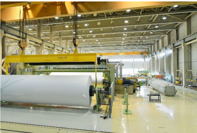
Figure 2: Steam is essential for paper production. (© Piller Blowers & Compressors)
