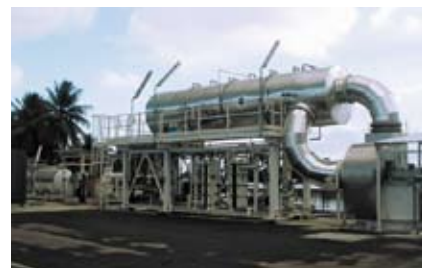
Vapour Compressor in a seawater desalination plant
