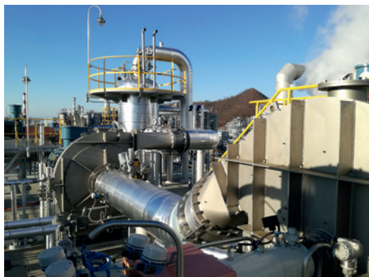
Fig. 6: Multi-stage system in operation
